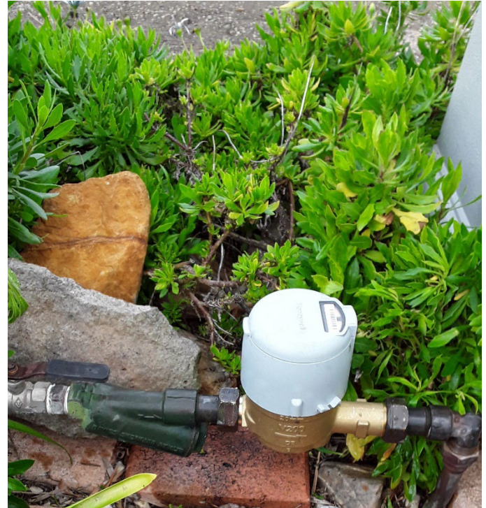
New smart water meters have been installed at properties across Narromine Shire Council.
